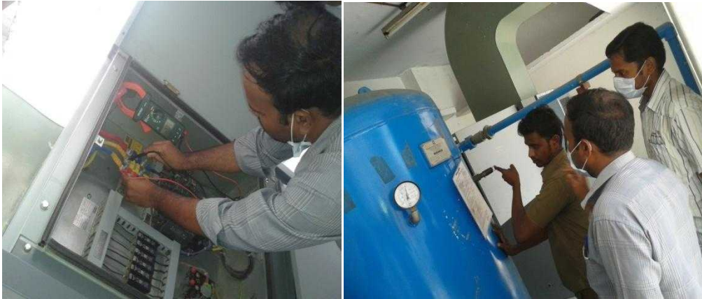
Fig. 2 Measurement of loading and unloading power in air-compressor
